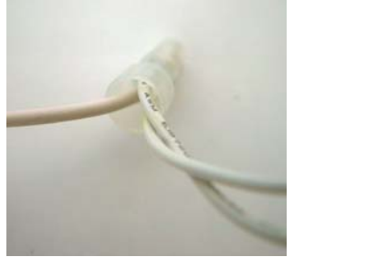
All white wires are connected together. The two from the transformer and the white - NEUTRAL from the power cord.
